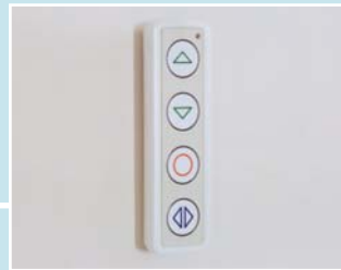
wireless landing controls
